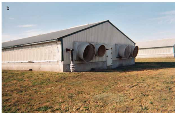
Figure 11.5. (a) Hybrid ventilation system with fans for cold-to-mild ventilation and curtains for warm-to-hot weather ventilation. (b) Hybrid ventilation system with tunnel fans for hot weather airspeed control.
